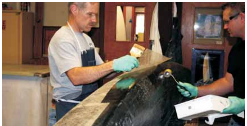
Pawlak and Ben Gougeon apply sheets of 1 oz/yd 2 fiberglass veil as an intermediate layer between the surface coat and the heavier mold laminate.
