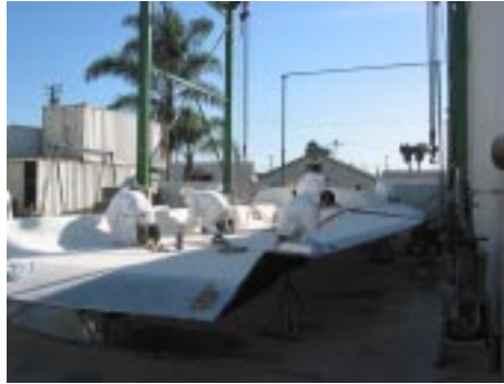
Alchemy deck construction - this isn't the photo we will be using - this is just for layout purposes.
